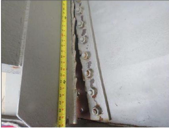
Crash damage on Bridge 230169 – 2023. The north side of the diaphragm is ripped loose.
