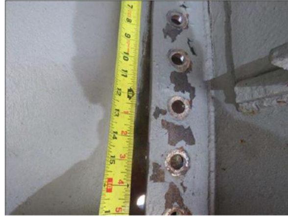
Crash damage on Bridge 230169 – 2023. Only 3 out of 10 bolts remained on the south side of Diaphragm 3.
