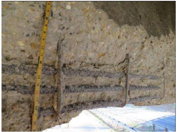
Crash Damage on Bridge 230106 – 11/23/21. Spalling with Exposed Rebar.
