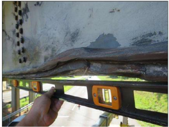
Crash damage on Bridge 230129 – 2021. Beam Out of Plumb.
