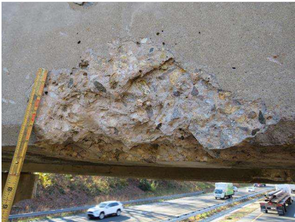
Crash Damage on Bridge 230106 – 11/23/24. Spalling.
